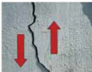
Uneven Loading and Settling of Footing
